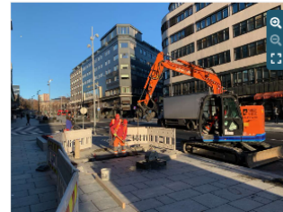
Workers put finishing touches to a novel 'zero-emissions' building site in central Oslo, November 2020 Photo: Alistair Doyle, Reuters
